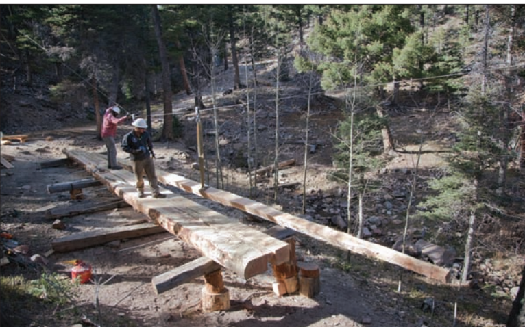
Conservation Department staff move a beam into place on Thurs., Nov. 1 at Cypher's Mine. The bridge, now completed, has been under construction since fall 2012. KATY MOONEY/PHILNEWS PHOTOGRAPHY MANAGER.
